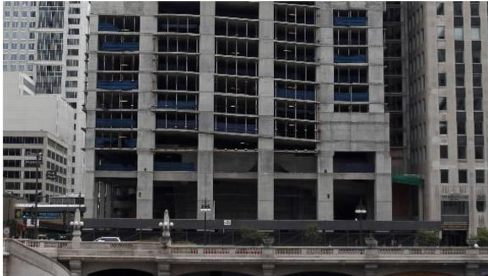
The 111 W. Wacker building is seen under construction in July 2011. (William DeShazer/Chicago Tribune / November 1, 2012)
